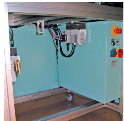
Switchgear cabinet and valve center
